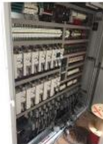
ELECTRIC CONTROL CABIN
